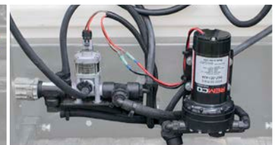
Electric pump and boom control
